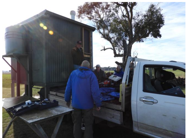
Murri's Ute made a convenient work platform to remove the iron sheeting and repair the broken pipe.
