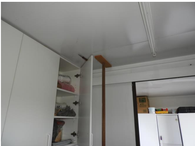
We had a problem with a section of the new ceiling lining where it bowed out and caught on the end door of the new cupboard when opened. I (Ed) drilled a few strategically positioned 4mm holes in the lining and squirted a 1/4 tube of
