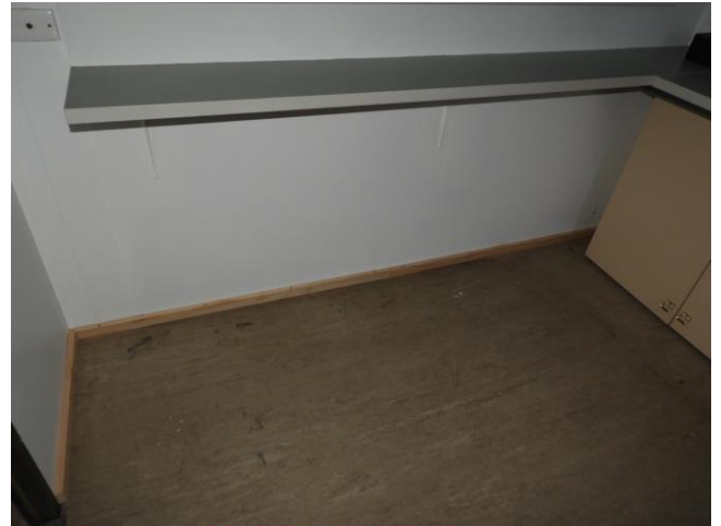
I (Ed) fitted a skirting board under the servery window on Sunday 16 th July – something we should have done years ago when the vertical door was removed and refitted horizontally to form the servery. The wall lining was a bit wobbly at floor level and lack of skirting to straighten it became more apparent once the kitchen had been painted.
