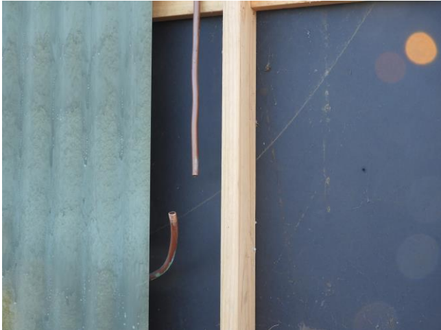
The 1/2 inch long split has been cut out so it can be re-joined. Pipework has now been lagged so hopefully it won't freeze and split again.
