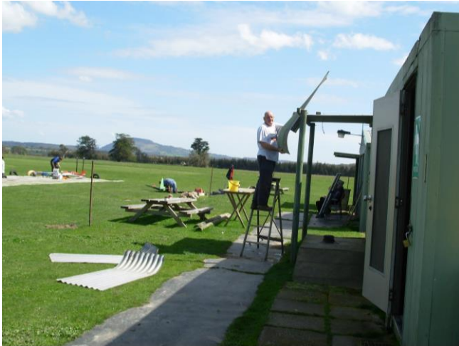
Sunday September 14 th . Dismantling the veranda over the servery in readiness to relocate the kitchen to hopefully Trawalla.
