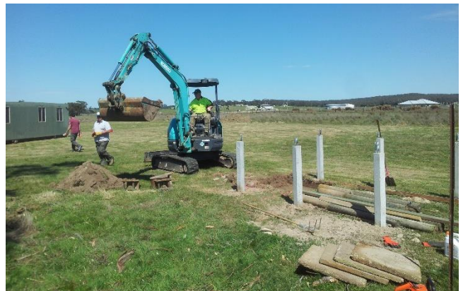
Martin Tuddenham's Kobelco digger was an invaluable asset during the day. Knocking down and digging out the tree marked for removal, hole for the composting toilet unit, dragging the old car away from under the big tree, it was going all day. Murri had set the concrete stumps in the ground a week or so prior to the working bee.
