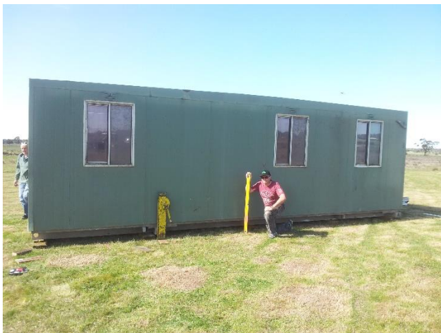
Trawalla jack in place. Noel with spirit level in hand was levelling the kitchen. The block is reasonably flat underneath sloping towards the door end.
