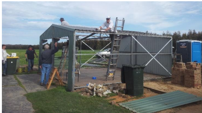
The shed came down quite easily in the reverse order of the original assembly. Fortunately we still have the assembly instructions and building permit info to assist with erection at Trawalla.
