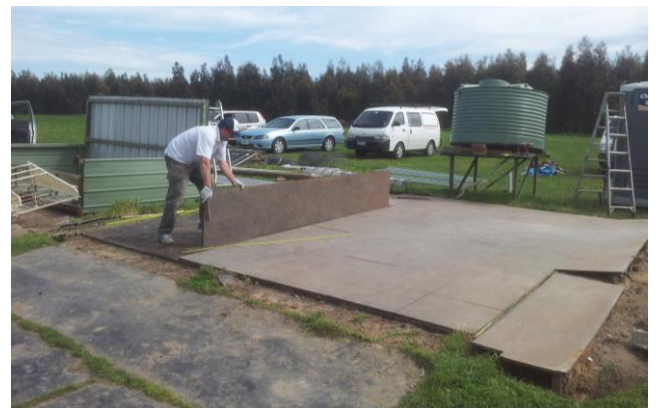
The flooring, a tongue & groove Laminex weatherproof particle board product was laid over crushed rock and packing sand with a black plastic membrane to keep the moisture out. It certainly has lasted and the intention is to reuse it at Trawalla.
