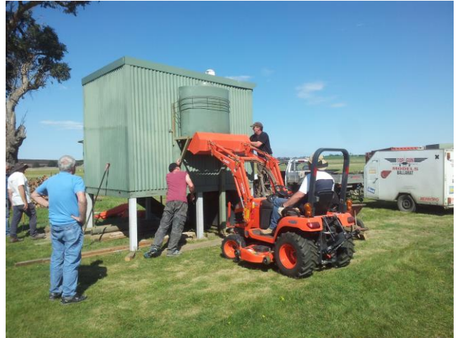
It did fit the foundations. Attaching the tank stand for the 500L tank. Graeme used his Kubota to hold it in place while the retaining bolts were attached. Concrete footings were then dugout and poured under the tank stand posts.
