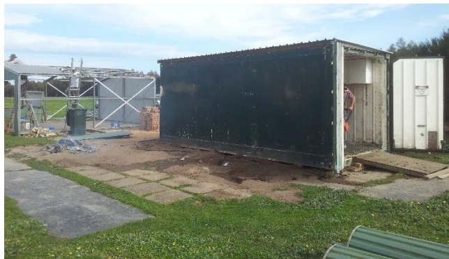
The shed was disassembled and all the parts packed up and loaded into the container. The particle board flooring which is quite heavy was spread out evenly over container floor.
