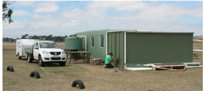
This shot shows the down pipes (there are two on the kitchen and one on each container) and the fill pipe going into the tank. (Photo taken on 11 th January.)
