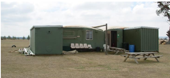
All the roof flashing has now been fitted which tidies up the new work considerably. (Photo taken on 11 th January.)
