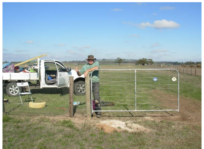
Murri Anstis fitted the two 2400mm gates in the fence that runs perpendicular to Church Road. Now it's the wet season, you don't miss the wet, muddy track that we had back at Spreadeagle Road and Spreadeagle Road got pretty muddy as well. Fortunately the 250m of Church Road which is unsealed has a high crown on it and stays reasonably firm.
