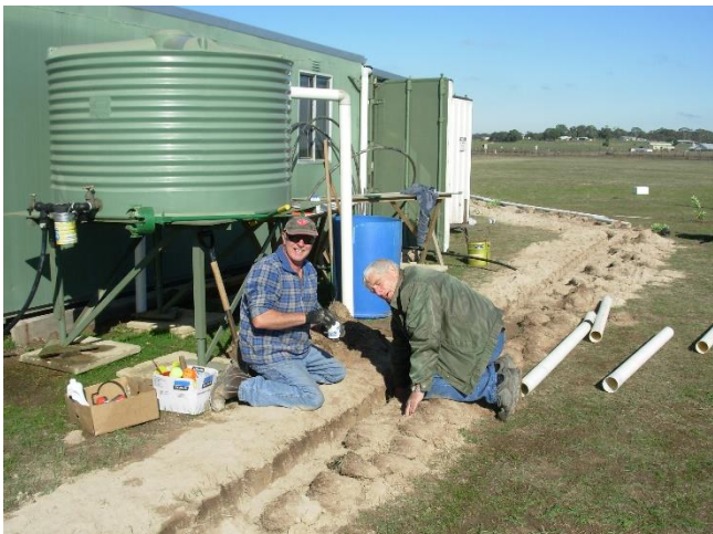
Wayne and Glenn working on laying the poly pipe in the trench. I hope those joints are water tight guys!!!
