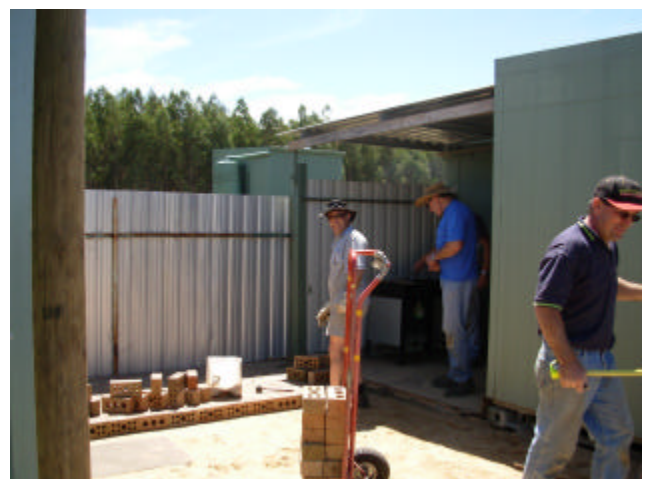
Half way through laying the bricks, Max has let us knock off for lunch.
