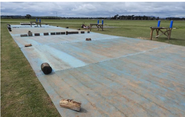
On Sunday 29 th September the matting was joined with a mastic adhesive. It seems to have stuck pretty well but we intend to put an adhesive strip over it to prevent it lifting with general traffic.
