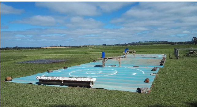
After a few hours work it was all in place ready to be joined and then trenched in. To prevent it blowing away, weights were place around the edge.
