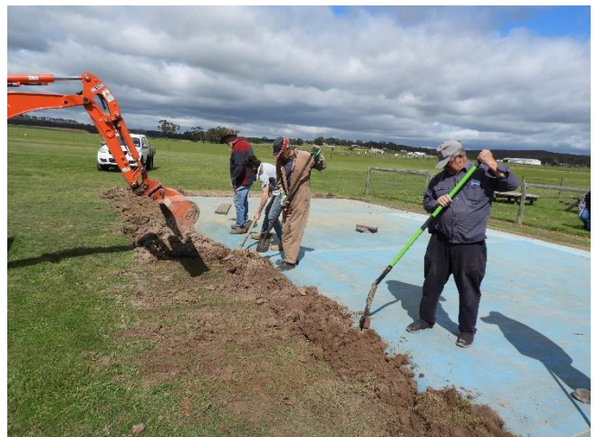
Backfilling was rather laborious. The digger helped push back the spoil, but with all the clumps of grass it was hard
