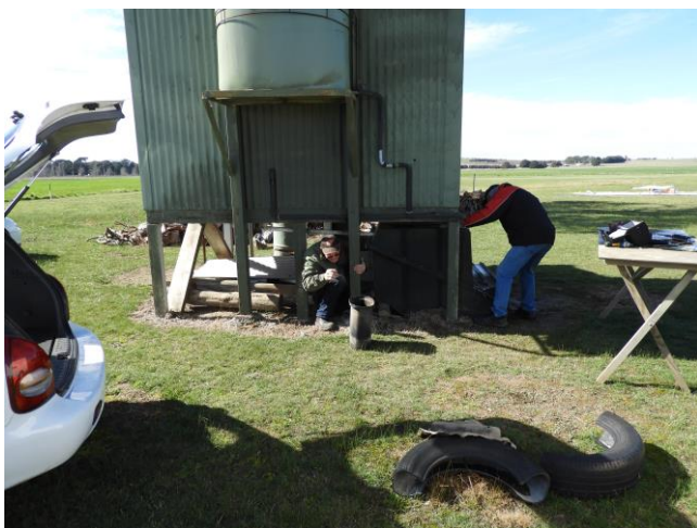
Max & Graeme working on fitting the new seal. Being right under the floor there's not much room to work.
