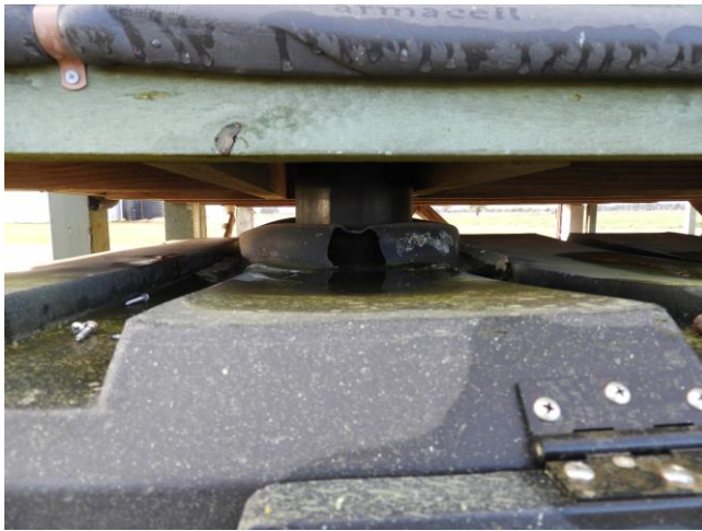
A section of the seal had disappeared recently leaving a gaping hole. The system doesn't work as it should if the seal is broken. It allows the wind to blow in venting inside making it a little smelly at times.
