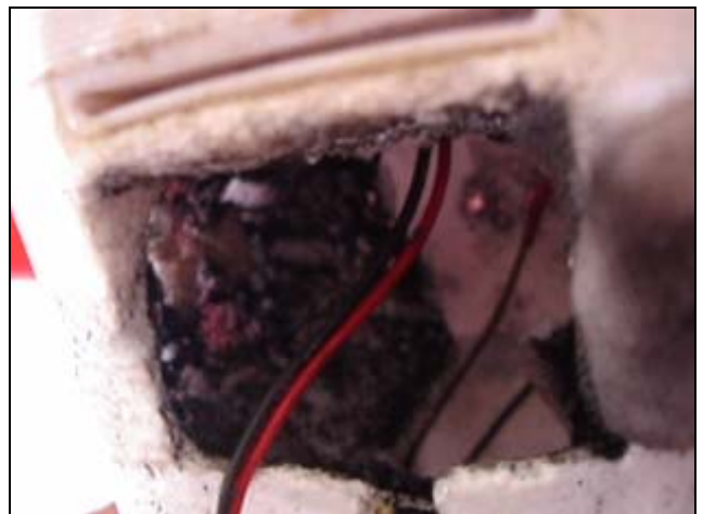
What was left of the battery bay; showing the charred polystyrene. Up to 2cm of foam was melted away.
